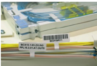
Fibre optic cable markers
