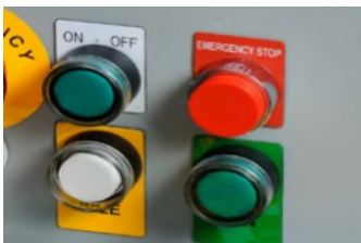
Control panel labels
